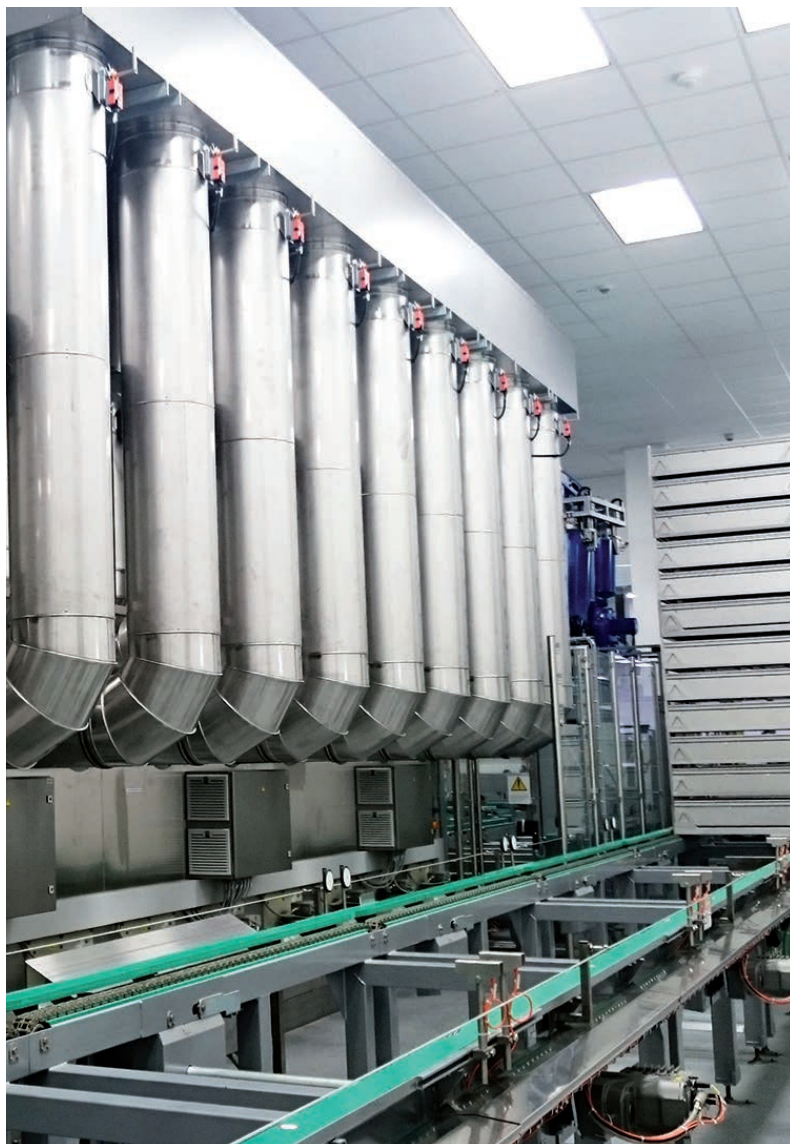
Cooling and drying tunnels are located downstream the sterilisers and operate alternately.
