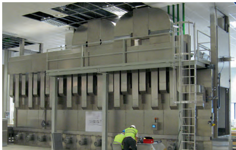
Fig. 2: Specially adjusted air ducting system between drying/cooling tunnel and dehumidification module. Insulation of piping prevents unnecessary heat loss.
