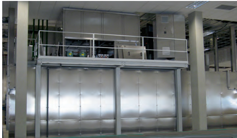
Fig. 1: Drying/cooling tunnel being installed. The attached AIRGENEX®med dehumidification module is placed on top of the tunnel to save space.
