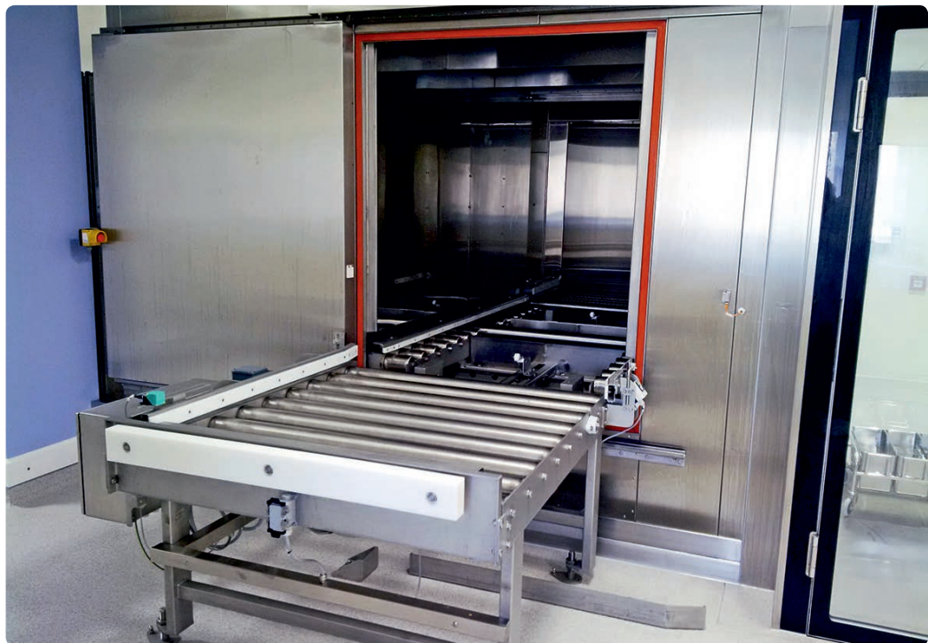
View into Drying-Cooling Chamber
