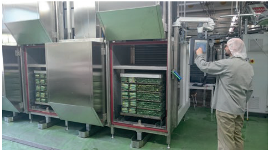
■ Fig. 3 – Packaged pasteurized sausage snacks are dried at 50 °C and then cooled to 38 °C in this batch dryer.
