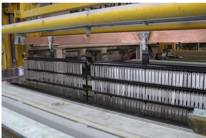
Rack upon entering the dryer subsidized in account of its energy efficiency (Photograph courtesy of Rudi Göbel GmbH & Co. KG)
