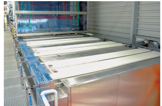
View of dryer in production operation
