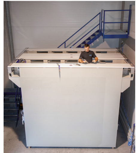
Engineer doing some welding work inside the impressively large new PP rack dryer (Photo: Harter GmbH)
