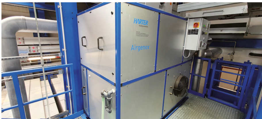
Insulated ducting connects the dryers with the Airgenex® dehumidification module which conditions the required process air. (Photo: Harter GmbH)
