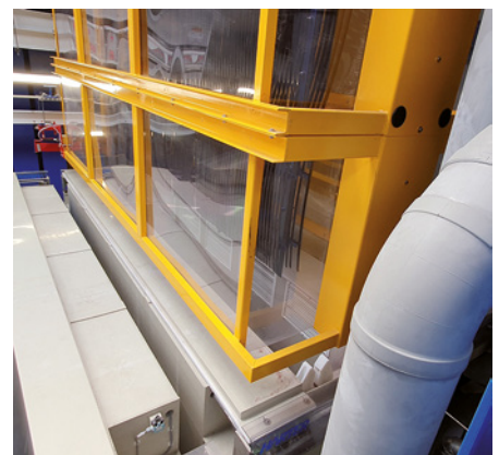
Carriage loading a rack into the dryer (Photo: Harter GmbH)
