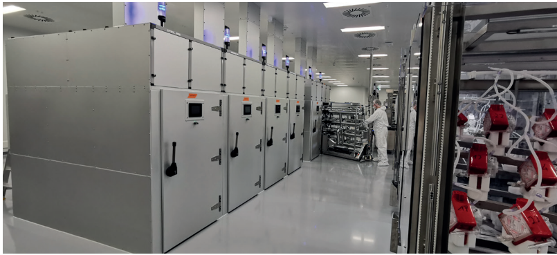
40 oxygenators each are processed in six identical dryers to become completely dry within 120 minutes at 48 °C maximum.
